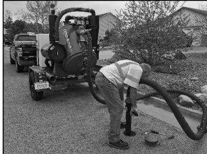
District team member Dana Stern cleans out a street valve box with the District's new vacuum excavator.
