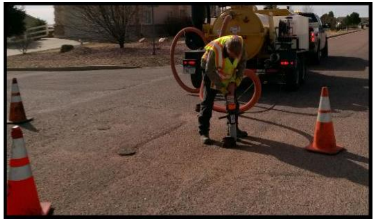
District Team Member Dana Stern performing a clean-out of one of the District's water main street valves at Liberty Grove and Cranston
